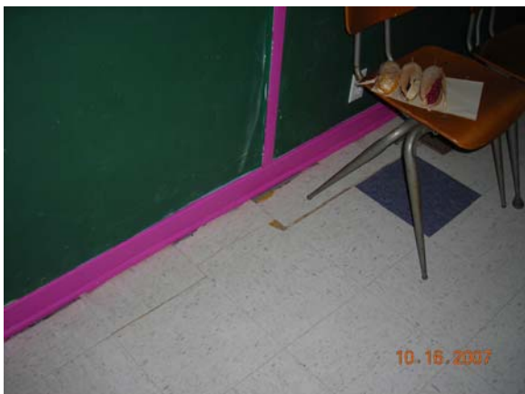
Photo 5 Wall Pulled Away
