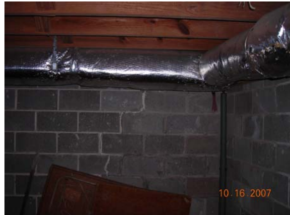
Photo 4 Foundation Wall Cracks
