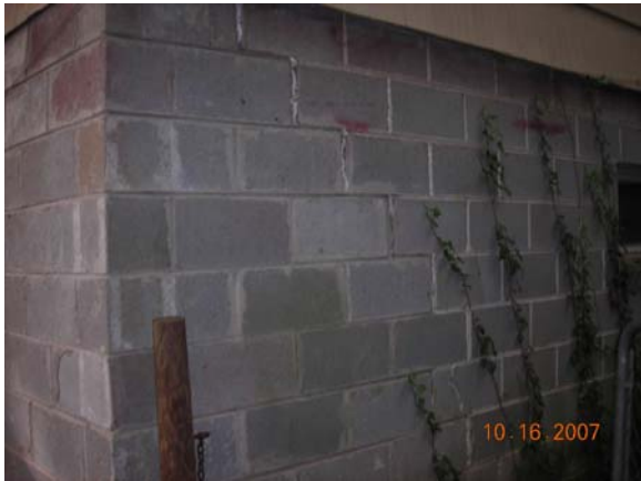
Photo 3 Foundation Wall Cracks
